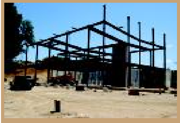
Pictured above is a photo of the Community Recreation & Environmental Center being constructed at Community Park in Haverford Reserve. For an update see page 5.
